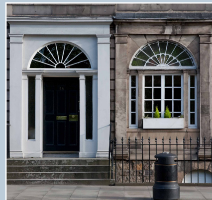
The old conversion of the right-hand doorway to a window and removal of the main entrance steps is disruptive to the character of the building and the broader pattern of entrances and windows in the street. © N. Haynes.
