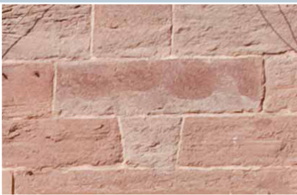
High Street, Arbroath. Rich pink-red sandstone, typical of parts of Angus. Here the stone is laid in regular courses. © N. Haynes.
