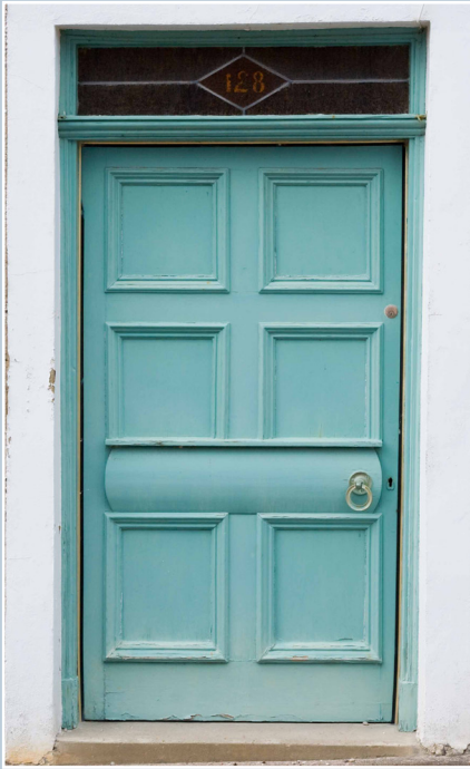
A timber panelled door in the Seatown at Cullen, Moray. The detailing of this door is typical of the high-quality joinery of the area. Draught-proof strips have been applied around the door. © N. Haynes.
