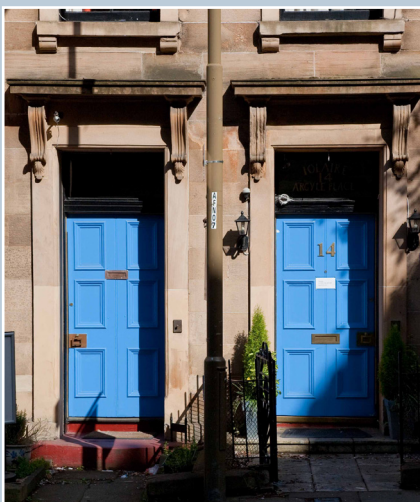
The door on the left is redundant following the internal amalgamation of two villas, but retained in place to maintain the character of the building. © N. Haynes.
